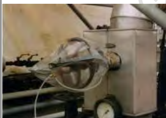
Figure 3.38: Bagging of a leaking valve
